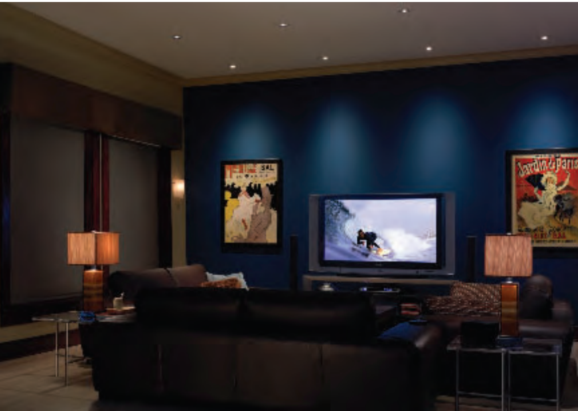
Lighting control immerses the user in the home theater experience, with lights that fade as the movie begins.
